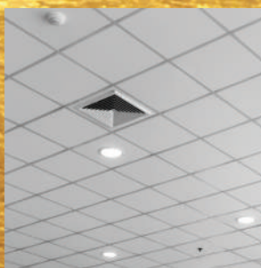
CEILING GRID FALSE CEILING
